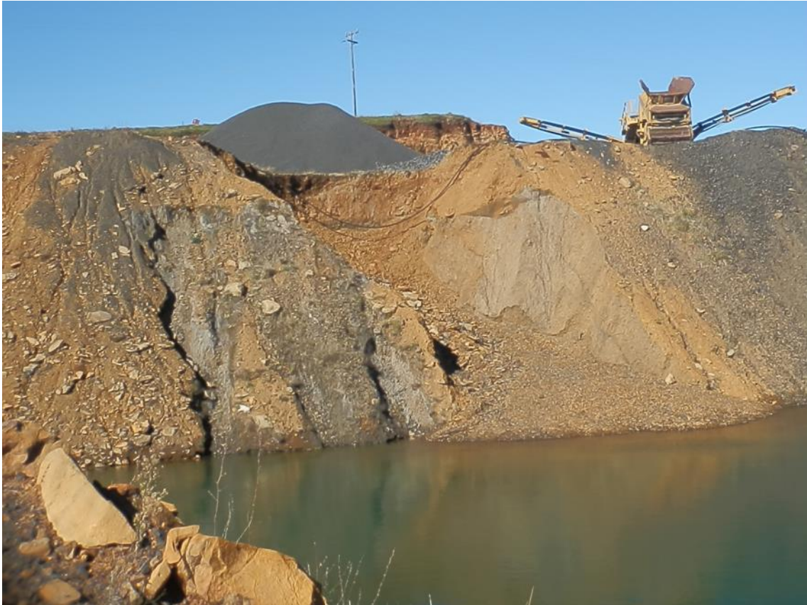
Plate 21: Alternative Site 4- Quarry Site - Close up view of the quarry face showing rutting erosion and minor instability (slumping).
