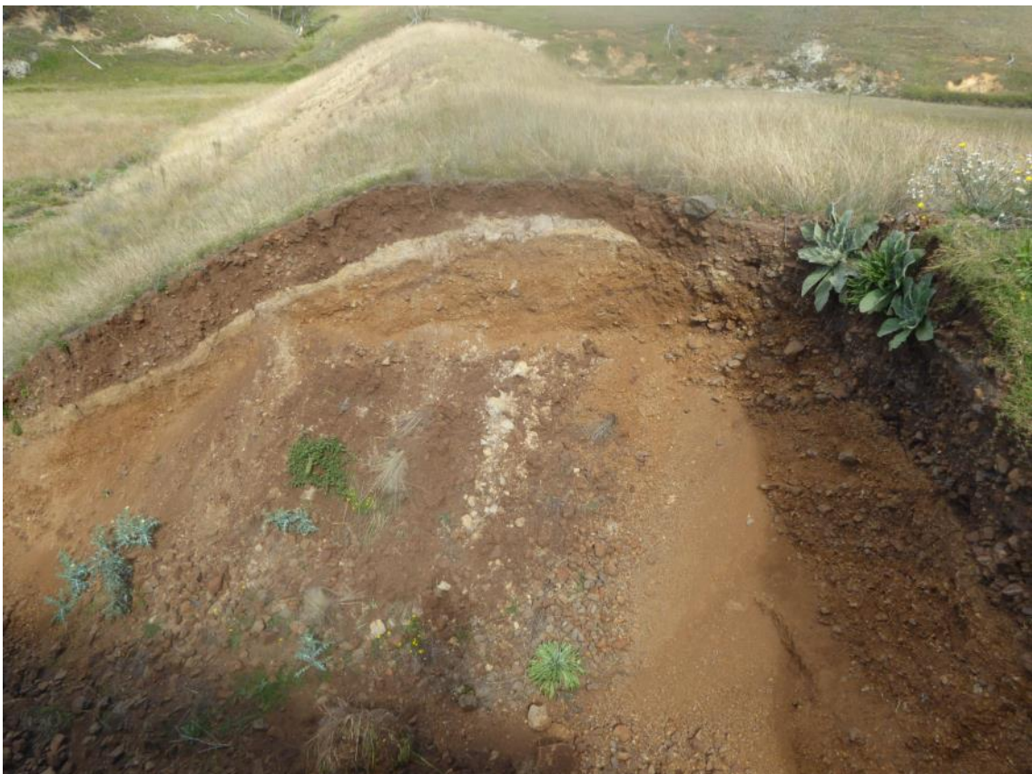
Plate 16: Alternative Site 3 Dam - View of the cutting at the north-western end of the existing right abutment.
