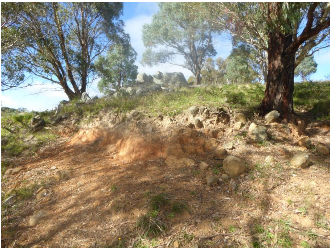
Plate 4: Guyra Dam 2 - View of the right abutment showing weathered basalt in the cut and basalt boulders on the ridge line.
