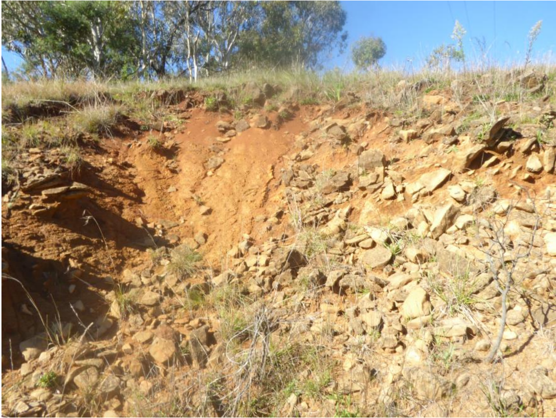
Plate 25: View of the rock cutting along the New England Highway, showing shallow residual profile.
