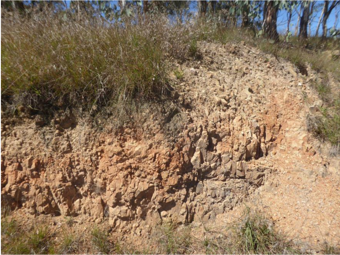
Plate 27: View of the cutting along the access road to Malpas Dam, showing highly to moderately weathered, highly fractured basalt.
