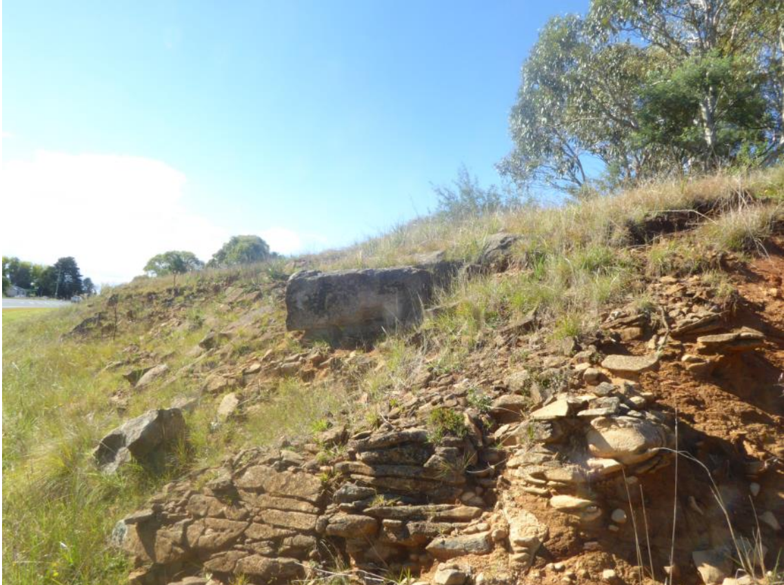
Plate 26: Another view of the above cutting showing variably weathered basalt. Note variable defect spacing with more massive outcrop in the centre.
