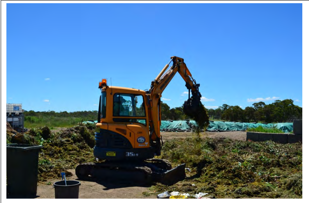
Photo 13. Spreading of the green waste organic waste in preparation for windrowing. Note windrows in background.
