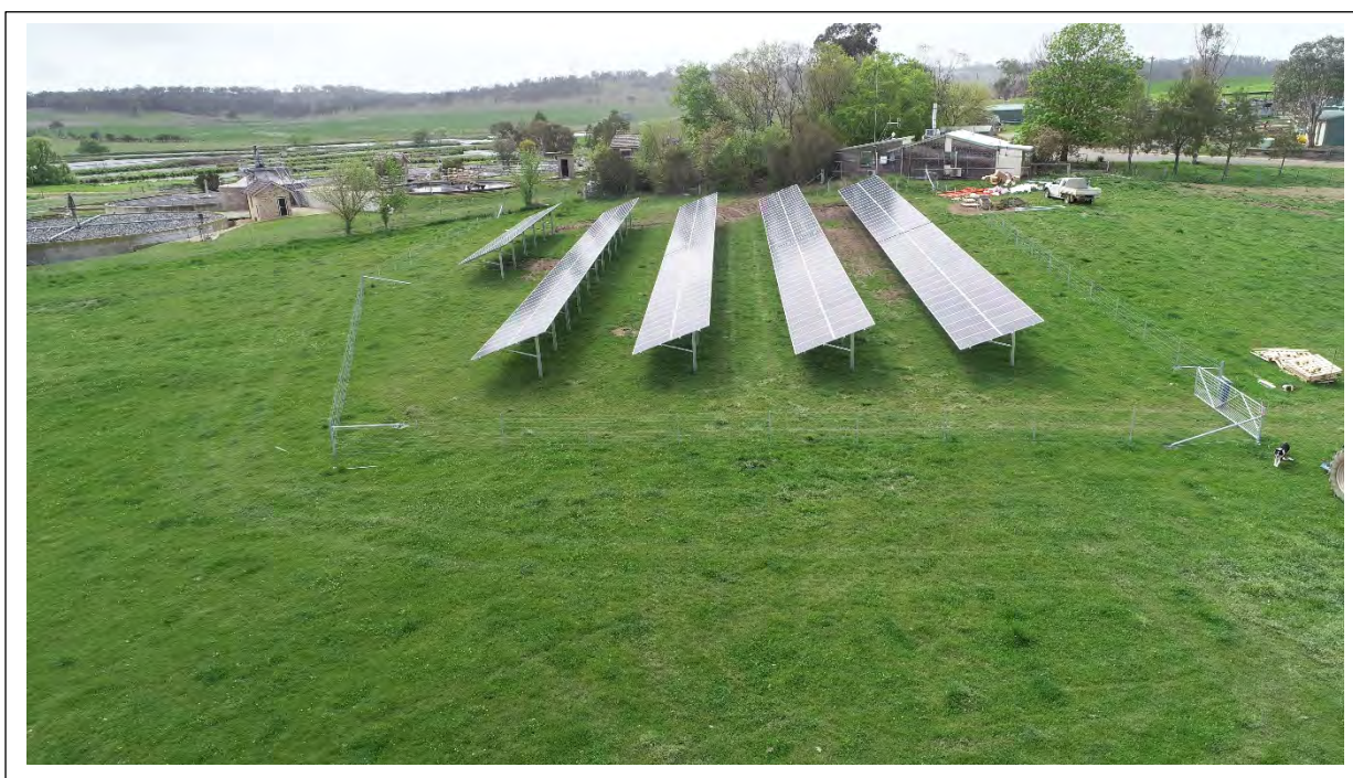
Photo 8. Solar installation at Wastewater Treatment Plant, 2018.
