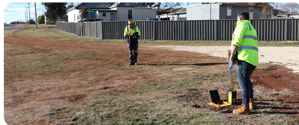
Specialist contractor Detection Services investigate the treated water network in Guyra for leaks
