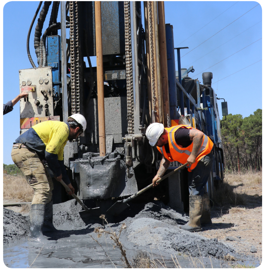
Contractor McKechnie Drilling undertakes test drilling at one of the potential bore sites on Rockvale Road.
