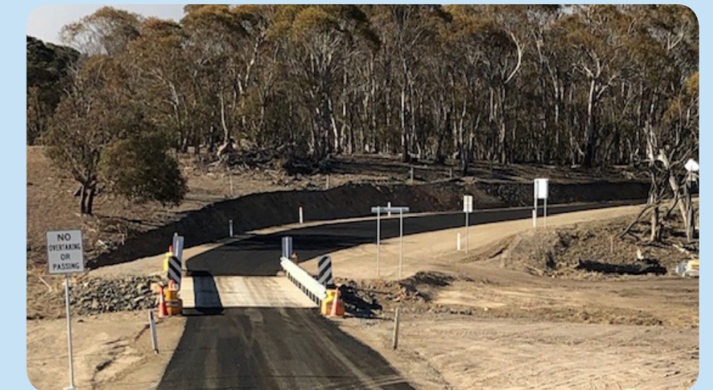
The Boundary Creek Bridge was one of two structures replaced by culverts on Rockvale Road as part of Bridge Renewal Program works in August.
