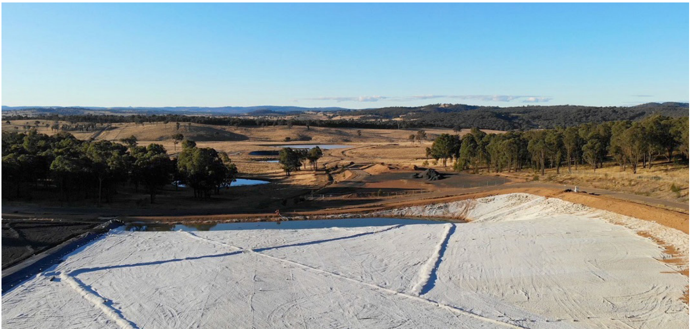
The first cell has been constructed and is divided into two sections to minimise leachate
