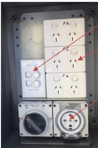
North power box
